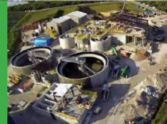
Cudjoe Wastewater Treatment Plant
